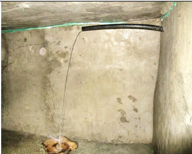
Pic. 24: The 25m 3 water storage tank is fully cemented on the inside, to prevent any leakage and to keep the water safe. The water flows from the spring through the ~1200 m long, underground buried, HDPE pipe into the tank
