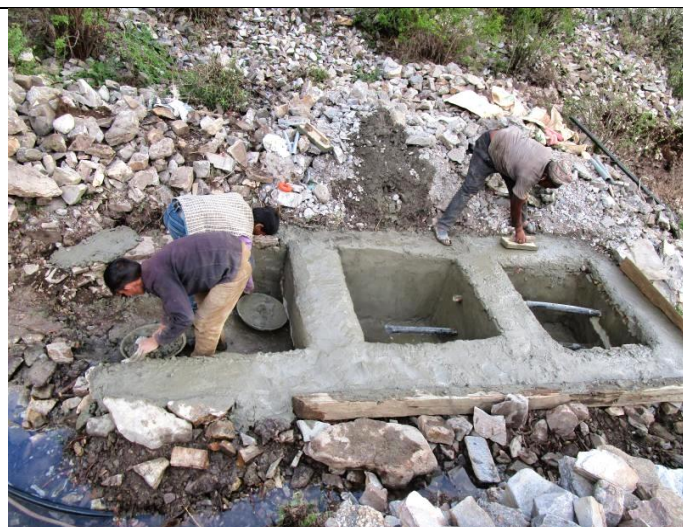
Pic. 17: The water source intake and sedimentation tanks with cement walls and cover to protect the source water
