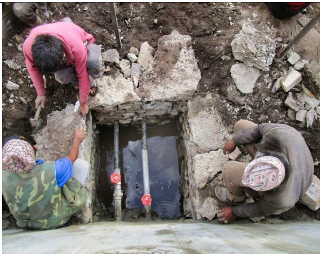
Pic. 26: The 25m 3 water storage tank is connected with four metal pipes, three of which are underground and one inside the tank respectively. From the water source, outlet to the 15-water tap stands in the village, overflow and for aeration. Here we see the outlet & overflow pipes, accessible for O&M
