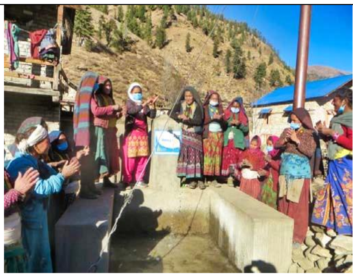
Pic.82: Pere women are using newly constructed DWS to learn proper hand washing
