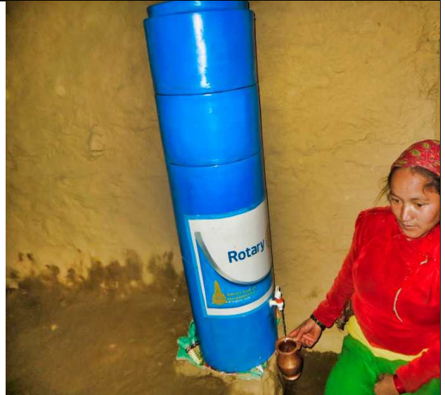
PIC.141. A Pere woman uses clean drinking water from the newly installed SSWF.
