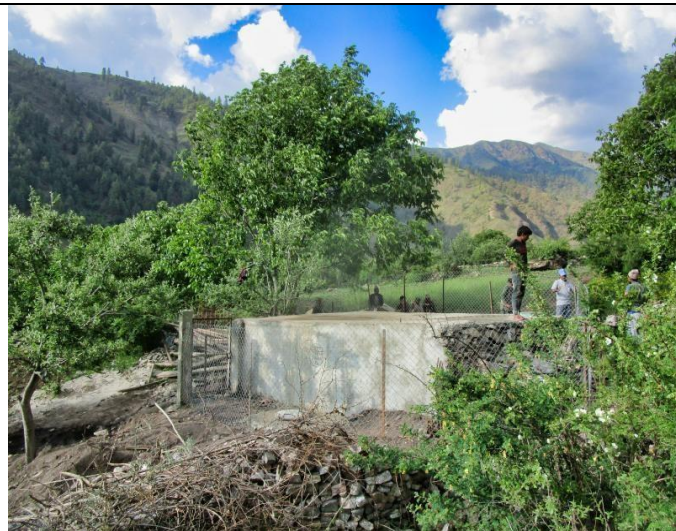
Pic. 25: In order to protect the drinking water from contamination by animals and people, the water storage tank is surrounded by a metal fence and a locked metal gate, with access for the operator only for maintenance
