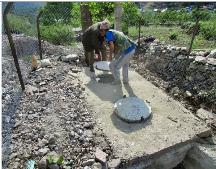
Pic. 18: The source water is collected in the cemented intake and sedimentation tanks, covered with a cement roof for best protection. Man-holes allow access to check and clean
