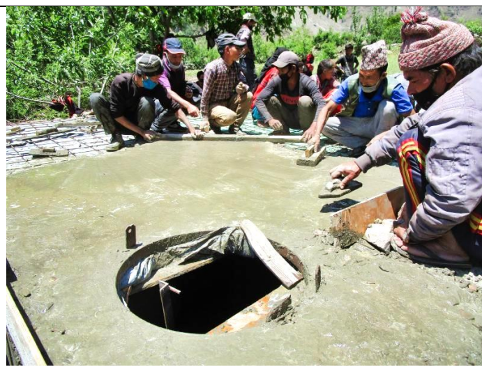
Pic. 23: In order to access the 25m 3 storage water tank a man-hole is integrated into the cemented cover lid. In this way the storage water tank is safe from contaminations and can be checked and cleaned periodically and easily
