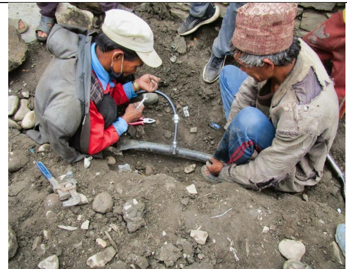
Pic. 27: The larger HDPE (High-Density-Polyethylene) pipe is the major pipe which is connected to the outflow metal pipe from the storage tank (Pic. 26) and going to all the 15 different water tap stands in the village. Here, a smaller HDPE pipe is connected to the bring water to one of the tapstands
